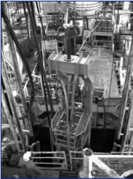
CT injection head hanging in the well-servicing derrick with CT reel behind.
